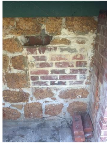
Figure 35 brick patch to wall behind condenser units
