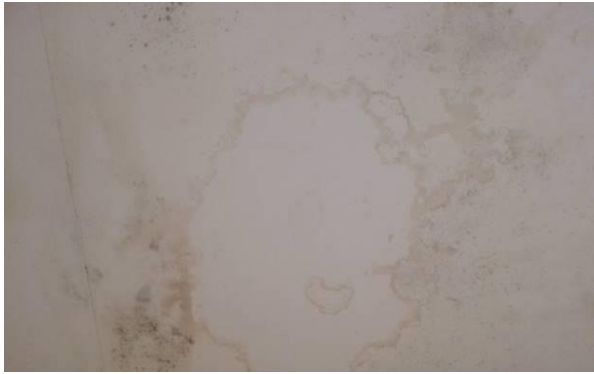
Figure 101 Water staining to ceiling of kitchen
