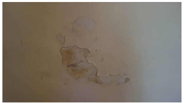
Figure 86 Evidence of damp bedroom 4
