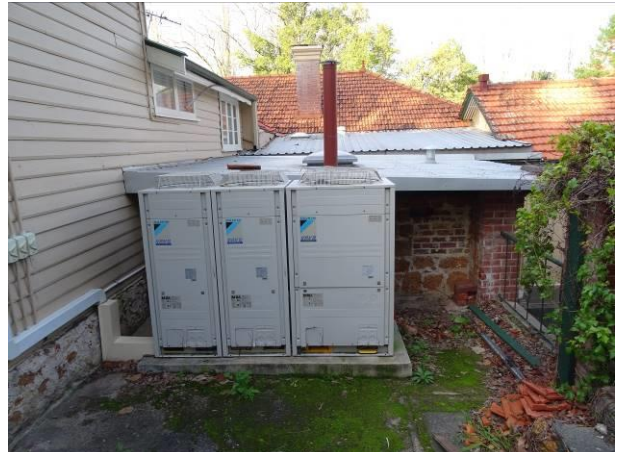
Figure 30 Condenser units to west
