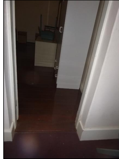
Bedroom 4 with limited circulation space to the latch side of the door
