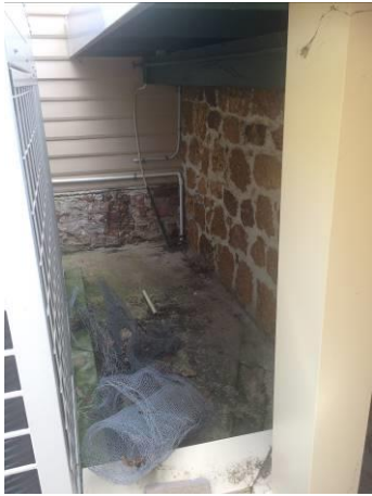
Figure 34 wall behind condenser units
