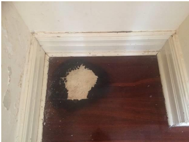
Figure 123 Bed 8, damaged floor
