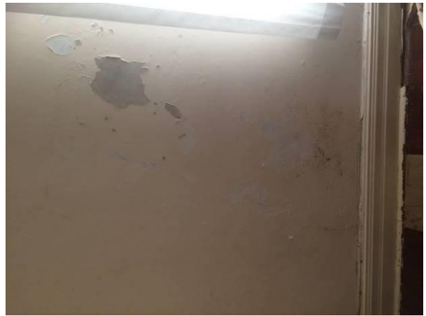
Figure 124 Evidence of damp to bedroom 8
