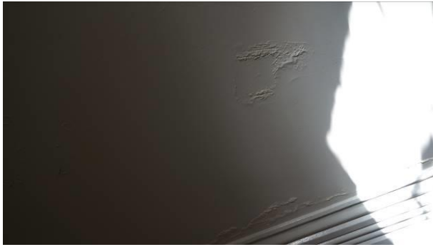
Figure 64 Main entry, evidence of damp
