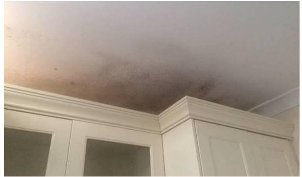
Figure 102 Water staining to ceiling of kitchen
