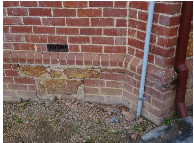
Figure 24 Fretted & damaged brickwork
