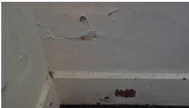
Figure 83 Evidence of damp to bedroom 3
