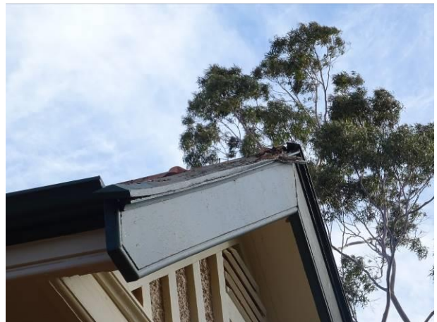
Figure 26 Damaged timberwork to gable end
