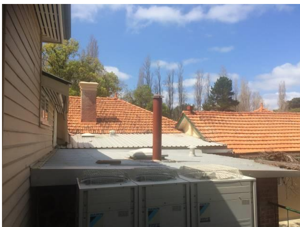
Figure 31 View over condenser units
