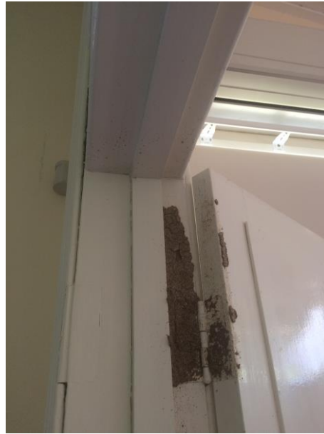
Figure 128 Sunroom, termite damage
