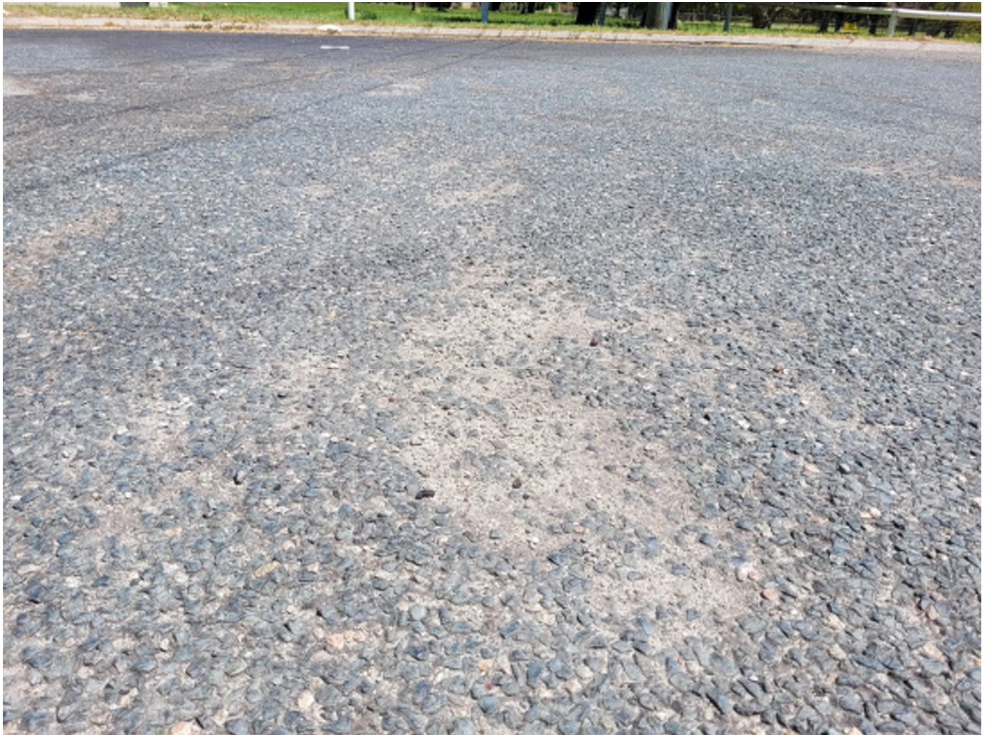
Photograph 6: Delamination noted near cul-de-sac along Hatch Court
