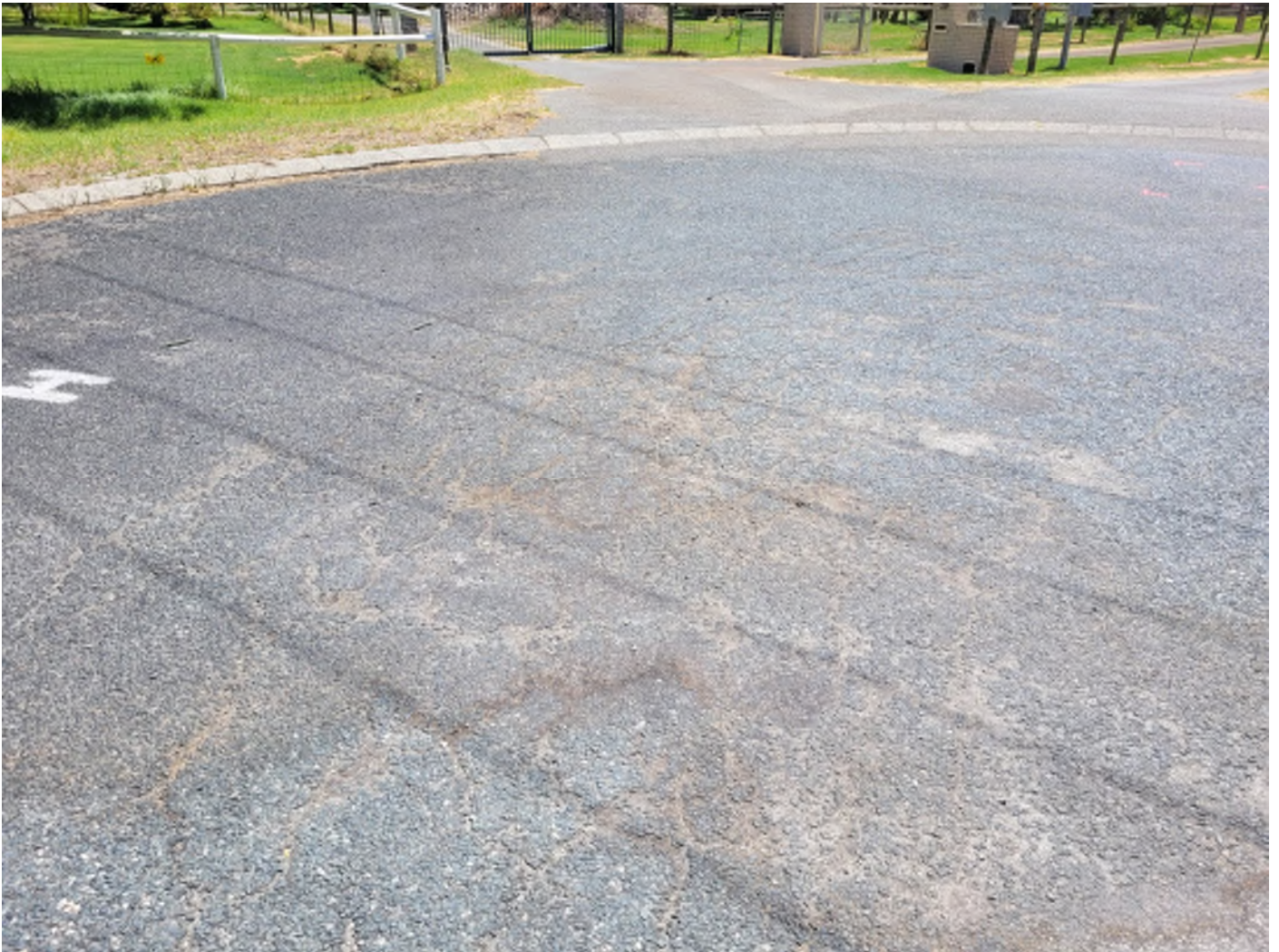
Photograph 7: Crocodile cracking noted near cul-de-sac along Hatch Court
