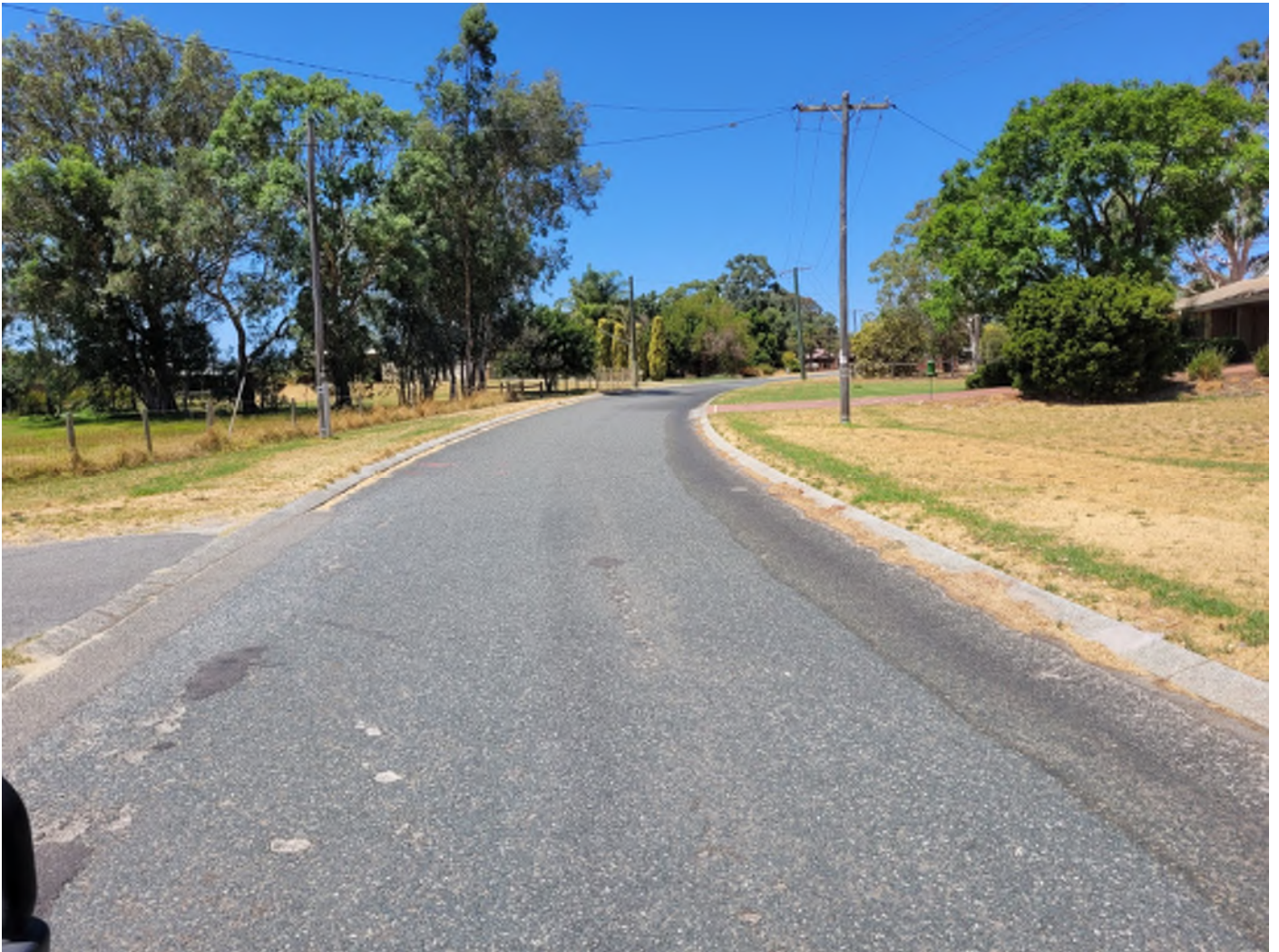
Photograph 8: Looking east from BH07 – minor delamination patches noted
